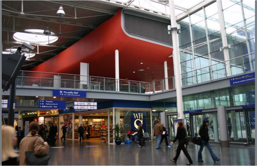
Piccadilly Station, Manchester. A combination of single and double bank louvres, depending on the specific airflow and rain defence requirements.
