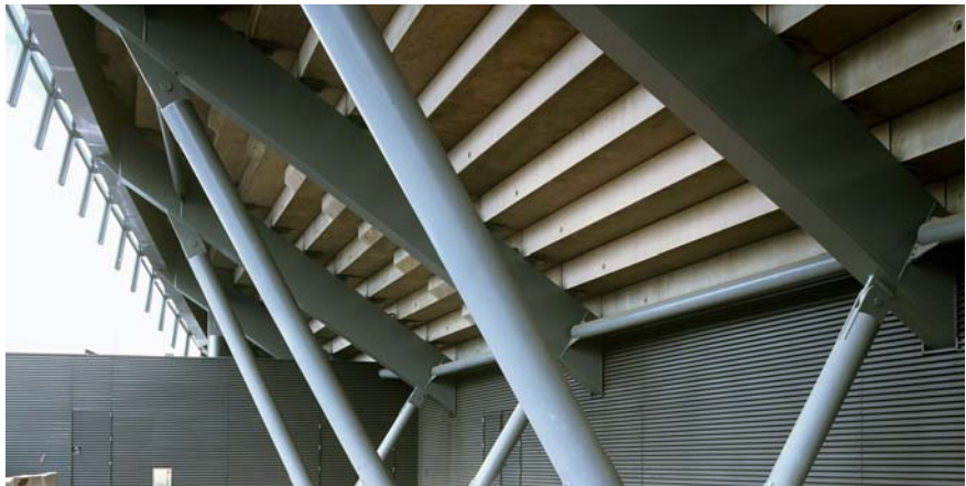
ERD rain defence louvre to plantroom enclosures.
