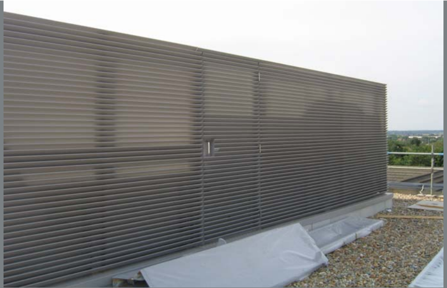
William Harvey Hospital, Ashford. IULISH inverted louvre panels.
