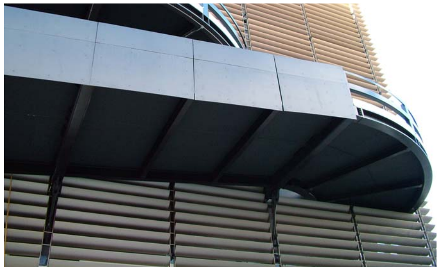
Paradise St Car Park, Liverpool Fixed Solarfin with special ladder mullion system and mitred corners.
