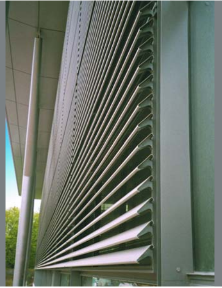
Clissold Leisure Centre, London. Vertical Solar C covers the glazing, which can be pivoted at an angle to facilitate easy cleaning of the glass behind.
